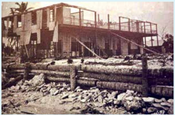
Figure 2-6. Typhoon Wind Impacts - Damage to the Catholic Girl's and Nuns' Living Quarters building in Jaluit after the 1905 typhoon. Note the blown off roof, which is common from the strong winds of a typhoon. In addition, there is water damage or inundation that overtopped the log seawall and eroded or scoured sediment behind the wall (Photo Micronesia Area Research Center).
