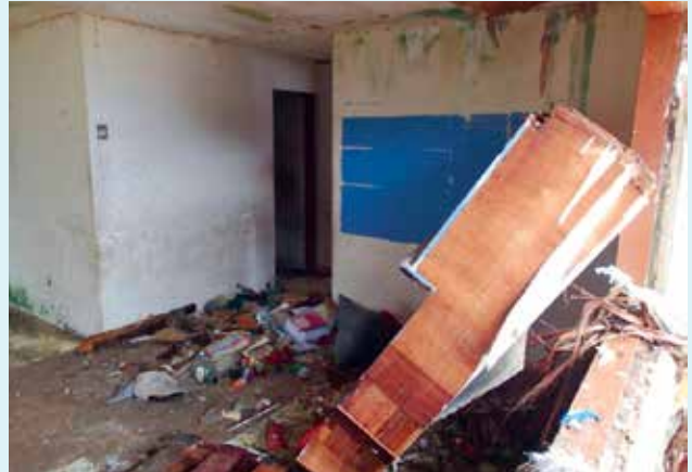
Figure 2-17. During the March 2014 event, about 110 homes were damaged and about 940 family members were displaced and sought sanctuary in government-designated shelters and churches. It is because of damage such as this that Part 4 of the handbook covers tools to reduce damage such as elevating of structures or building with flood resistant materials.
